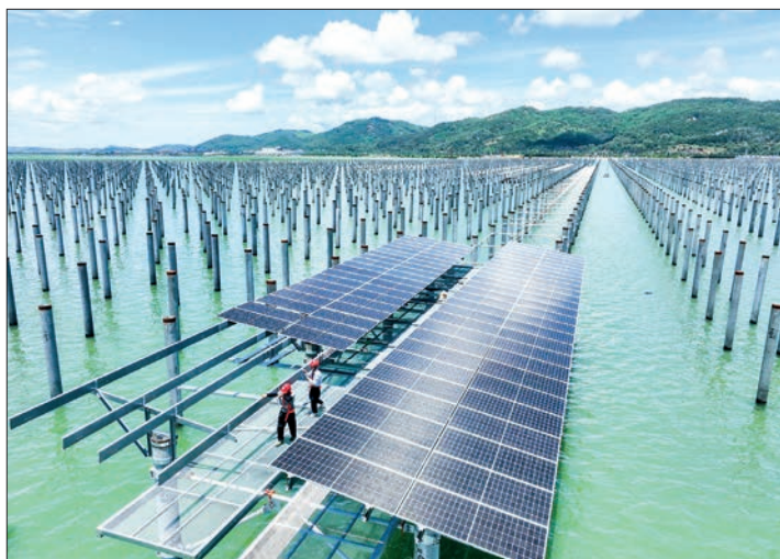
In this undated file photo, technicians install photovoltaic panels at a solar power farm in Dongshan county, Fujian province. PHOTO: XINHUA
