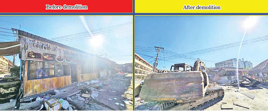
An illegally constructed single-storey residential building in KK Park Area (Section 3).
