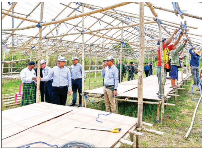
Kachin State Chief Minister U Khet Htein Nan inspects the construction of housing for IDP in the RC compound in Makhawyan Village, Waingmaw Township, yesterday.
