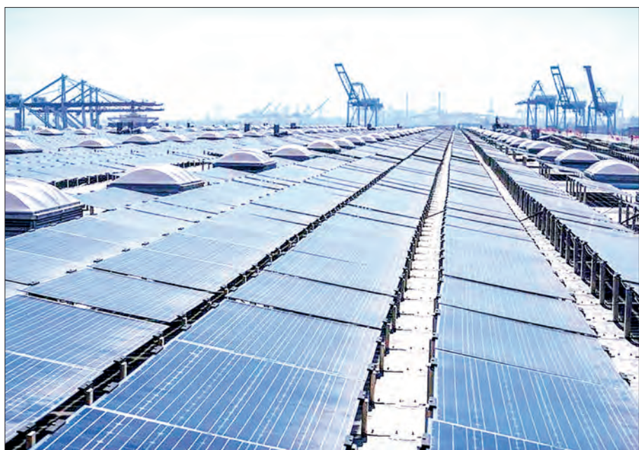
Photo taken on 26 June 2017 shows the 16.4 Megawatt (DC) Westmont Solar Energy Project in San Pedro, about 40 km south of Los Angeles, the United States. PHOTO: ZHAO HANRONG/XINHUA
