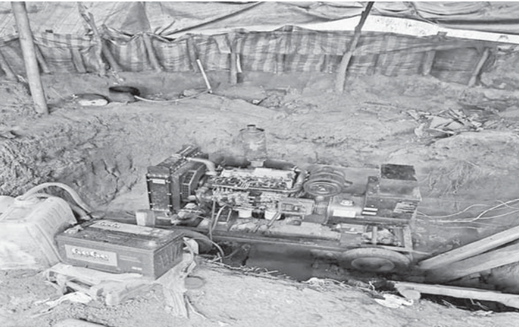
Record photo of a medium-sized generator.
