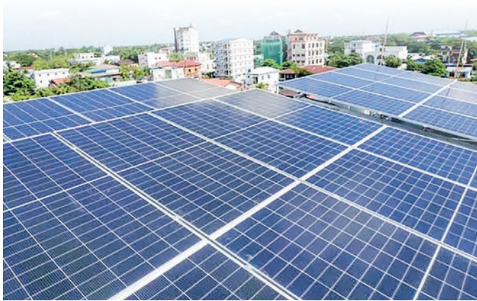
This picture shows solar power being installed at the rice mills in the Thilawa Special Economic Zone.
