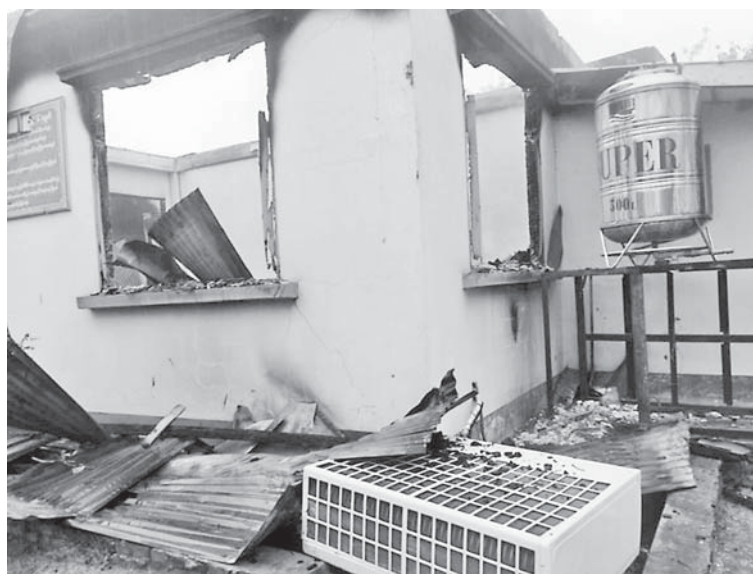
Photo shows damage to the vest factory in Taungtha Township after PDF terrorists set the factory ablaze.
