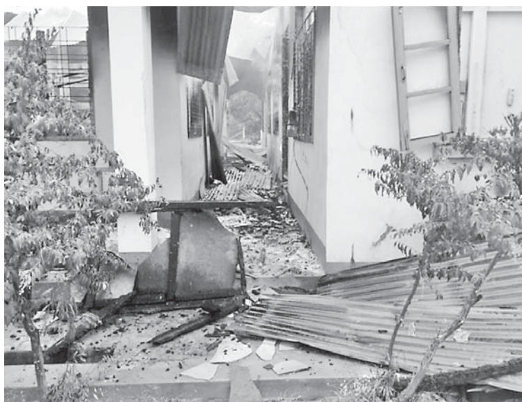
Photo shows damage to the vest factory in Taungtha Township after PDF terrorists set the factory ablaze.
