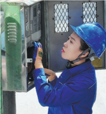
Meng Yuan examines electricity meters in Guang'an, Sichuan.
