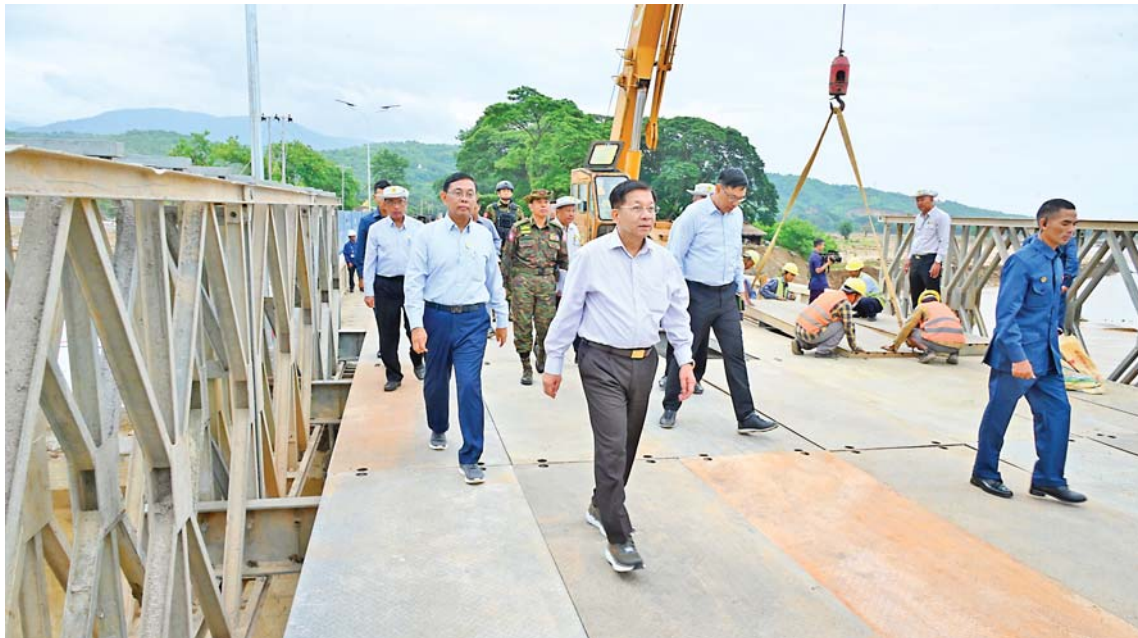
Senior General Min Aung Hlaing inspects construction of a temporary bridge across Nawin creek.
