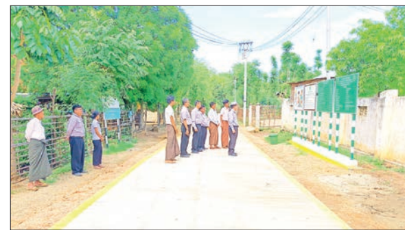
Officials inspect the completed status of the village concrete road in Minbu Township, Magway Region.
