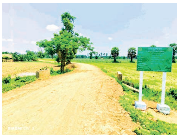
This image displays the completion of the rural production road in Lewe.
