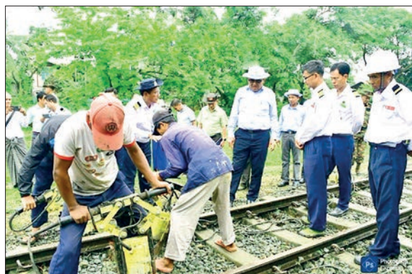
Railway tracks in Kachin State are currently repaired around the clock to enable the resumption of the Myitkyina-Mohnyin train service in July.
