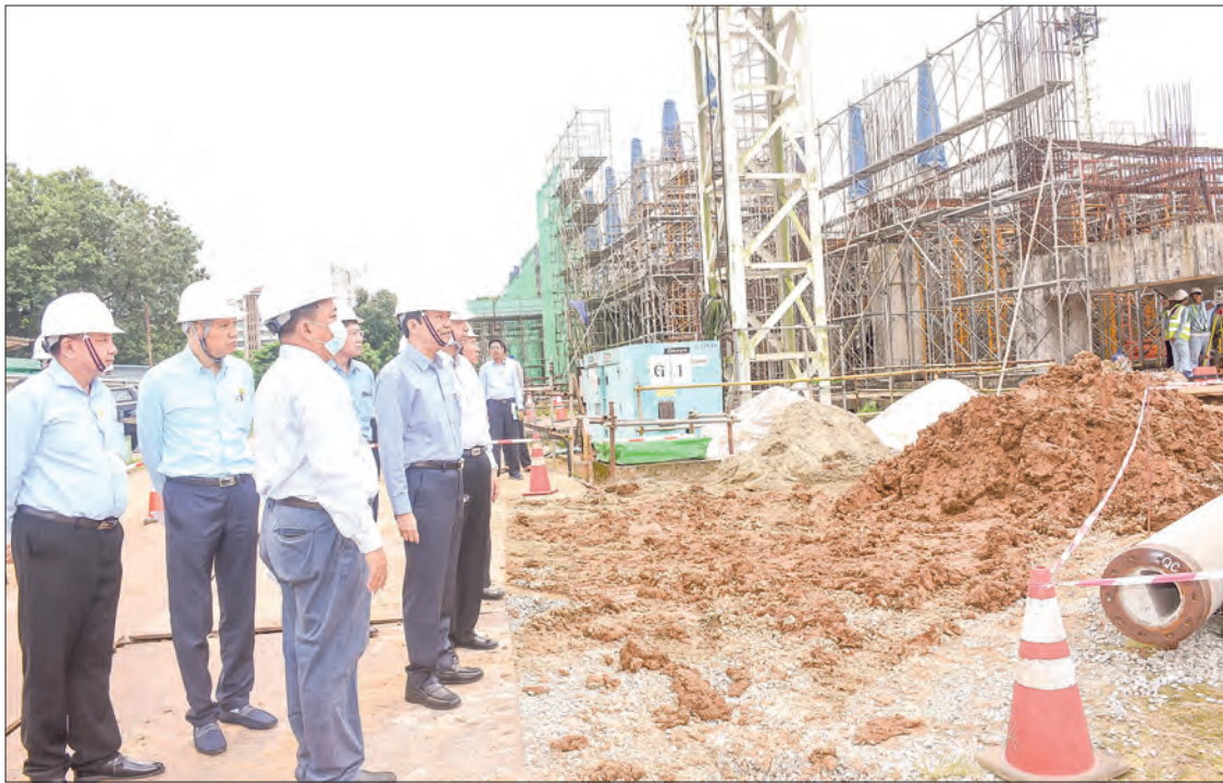
Union Minister for Health Dr Thet Khaing Win looks into the progress of the construction of New Yangon Specialist Hospital project in Lanmadaw, Yangon on 5 October 2024.
