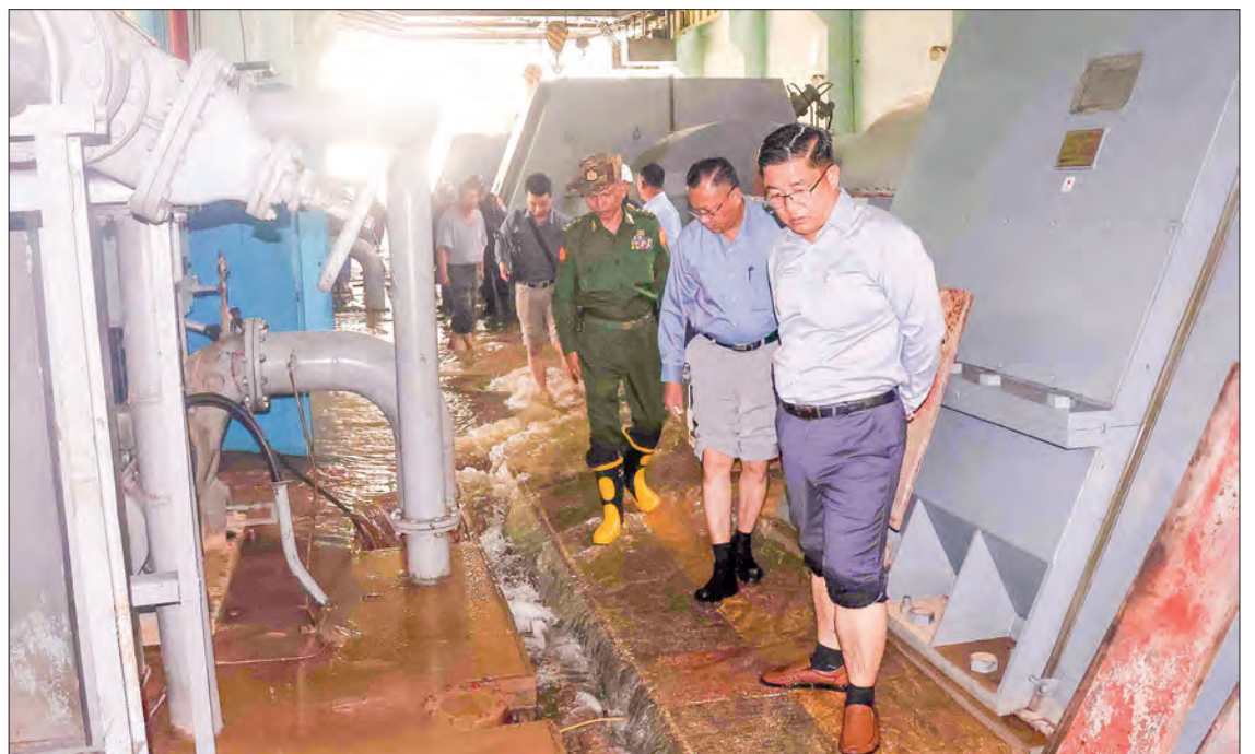
Kayah State Chief Minister U Zaw Myo Tin looks into the ongoing water removal operations inside the No 2 Biluchaung Hydropower Plant (Lawpita) yesterday. PHOTO: KAYAH STATE IPRD
