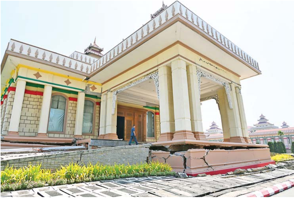
Damage at the Hluttaw buildings.
