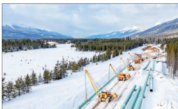
This 9 December 2021, image courtesy of Trans Mountain Corporation shows pipeline construction work in Valemount, British Columbia, Canada. PHOTO: HANDOUT / TRANS MOUNTAIN CORPORATION/ AFP/FILE
