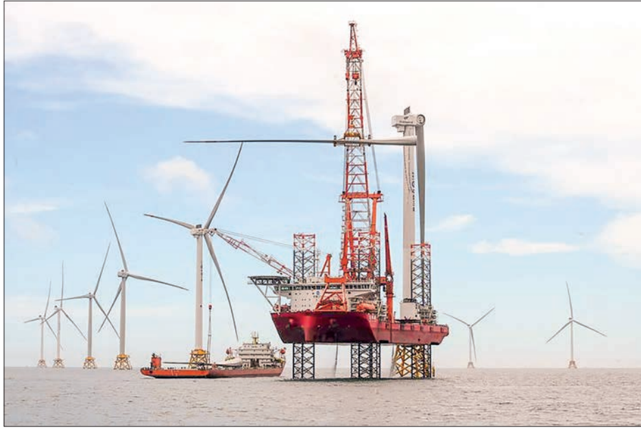
This photo taken on 19 June 2024 shows workers installing the blade of a 16-megawatt wind turbine of the phase II project of Zhangpu wind farm in southeast China's Fujian Province. PHOTO: XINHUA
