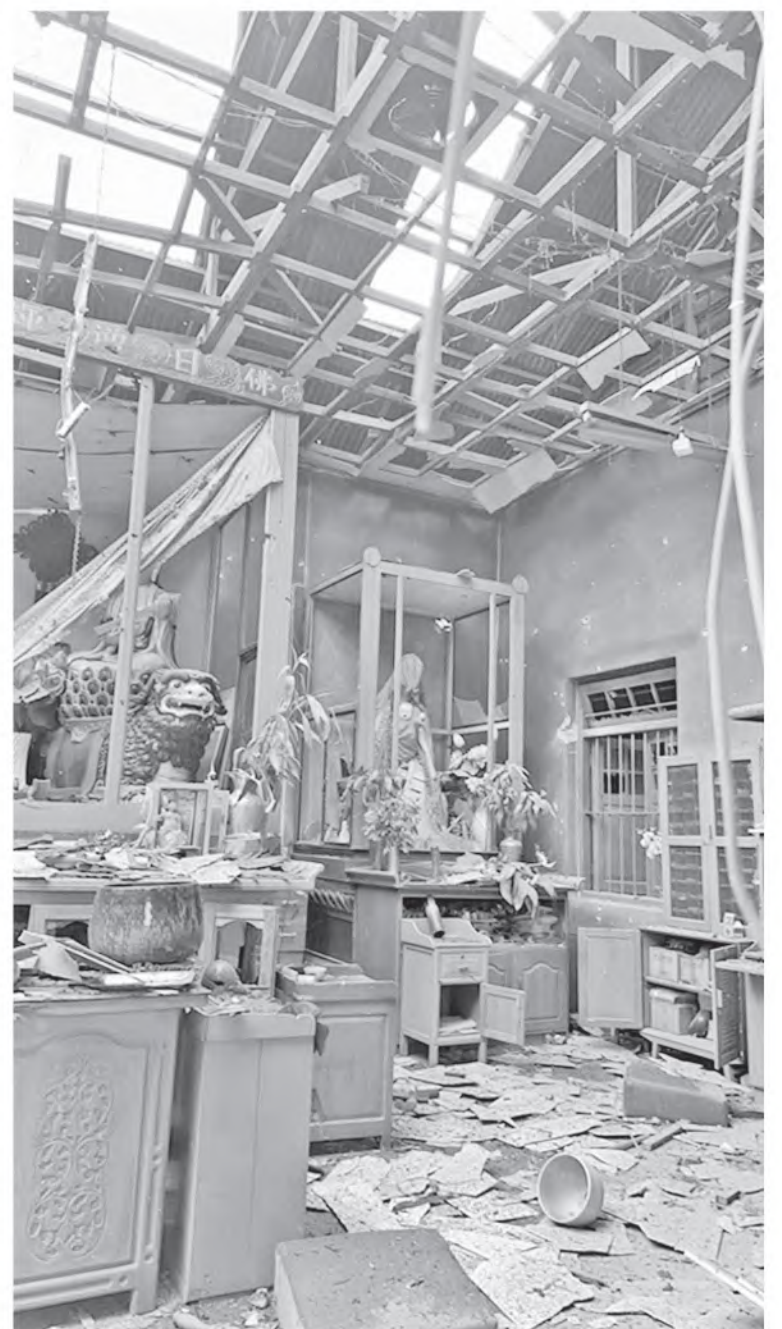
Photo shows the sector of Chinese temple destroyed by drone and drop bomb attacks of MNDAA.
