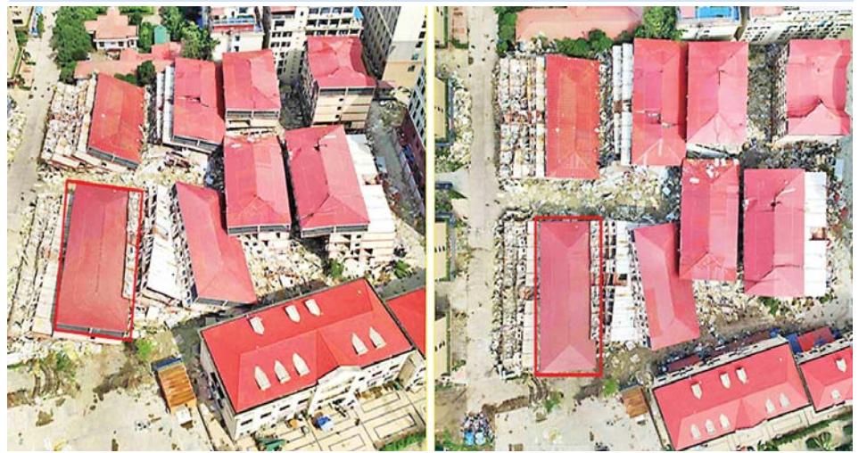
The illegal seven-storey residential building in the Shwe Kokko Area, Myawady District, Kayin State, where online scam gambling operations were conducted, has been destroyed with explosives.
