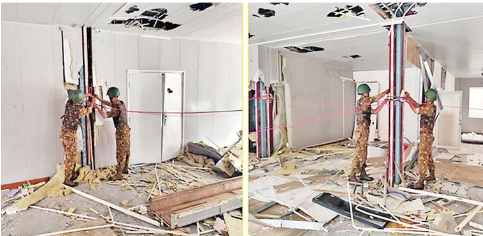
Preparation to destroy the illegal seven-storey residential building in the Shwe Kokko Area, Myawady District, Kayin State, where online scam gambling operations were conducted, using explosives.
