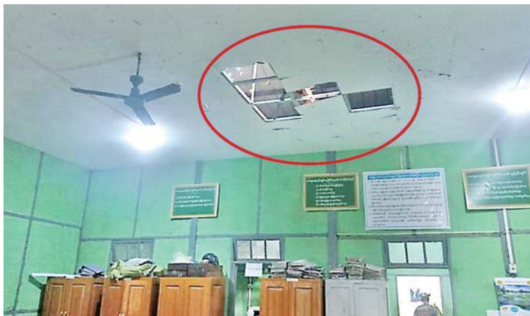
Damage caused by terrorist drop bomb attack on the Htantabin branch of the General Administration Department.
