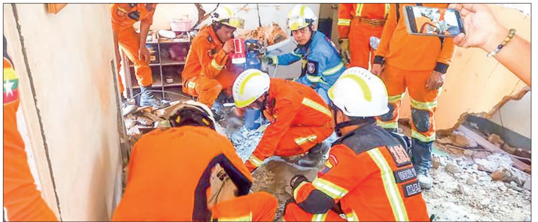
Firefighters are struggling to save a 62-year-old government retiree from the debris.
