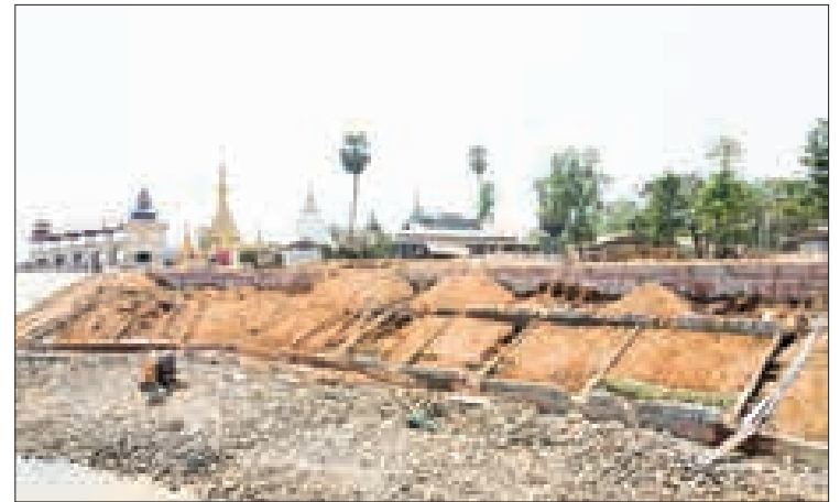
This photo depicts preparation works being launched to prevent the bank from collapsing due to river erosion.
