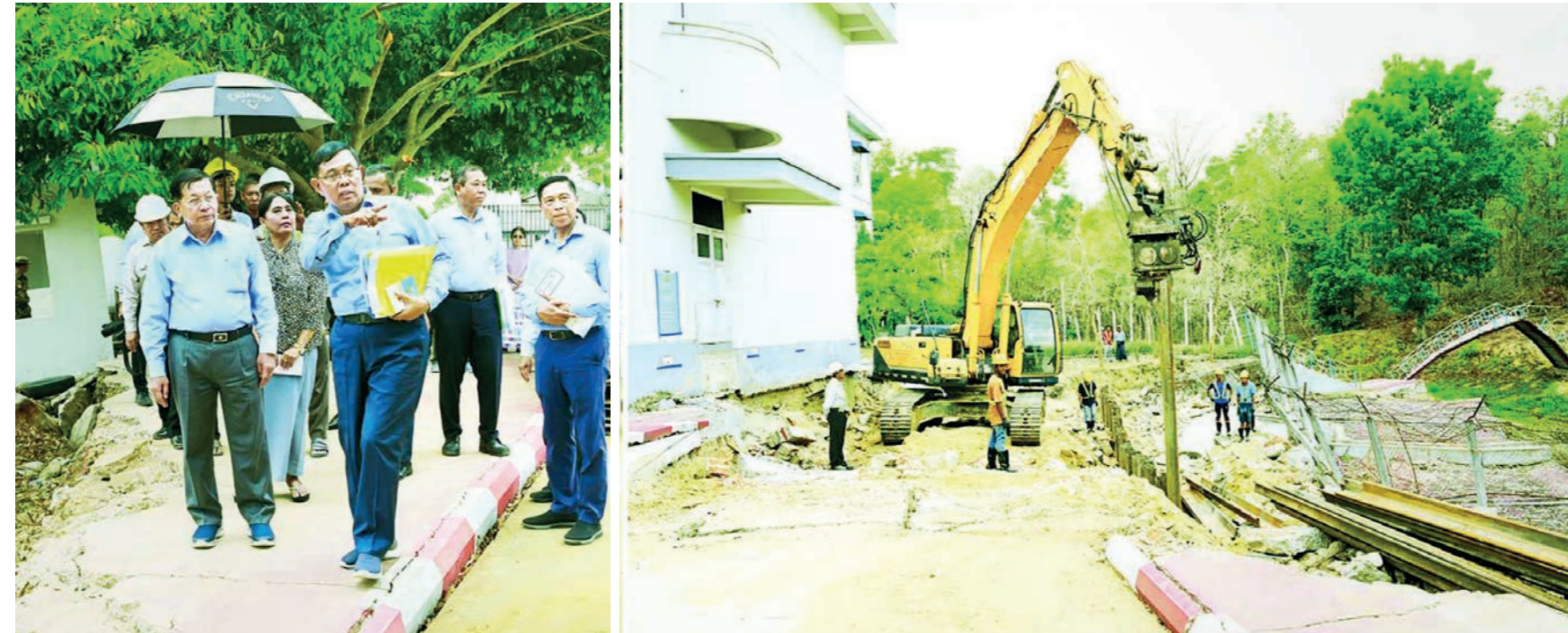
State Administration Council Chairman Prime Minister Senior General Min Aung Hlaing inspects the collapsed retaining wall at the Ministry of Legal Affairs, which damaged by Mandalay earthquake.
