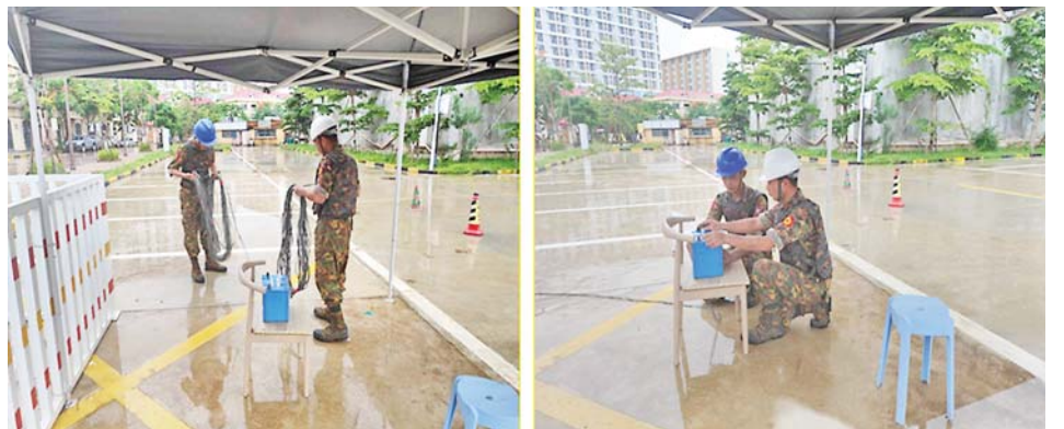
Preparation to blast and destroy with explosives an illegal seven-storey residential building where online scam gambling operations were conducted in the Shwe Kokko area of Myawady District, Kayin State.
