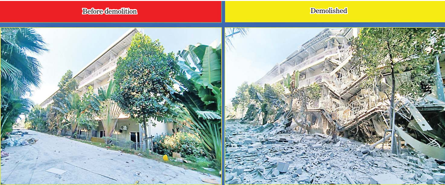
Illegally constructed four-storey building No. C 1 residential building in KK Park Area (3) (7.12.2025).
