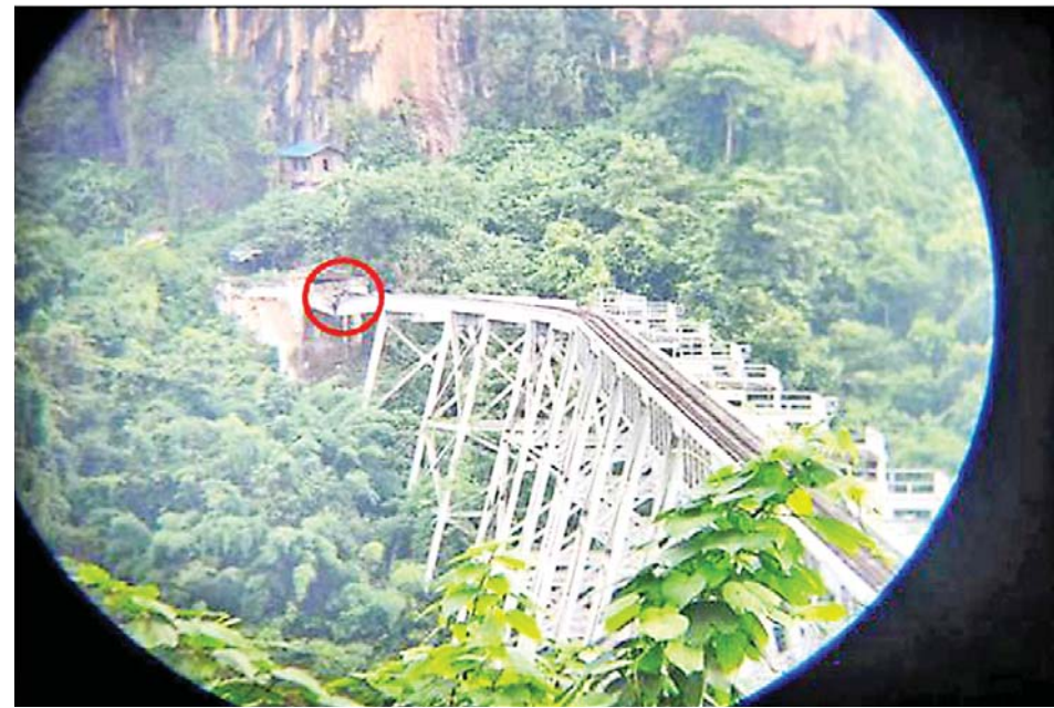
Damage caused by TNLA terrorists planting and detonating mines to destroy the Gokteik Bridge.
