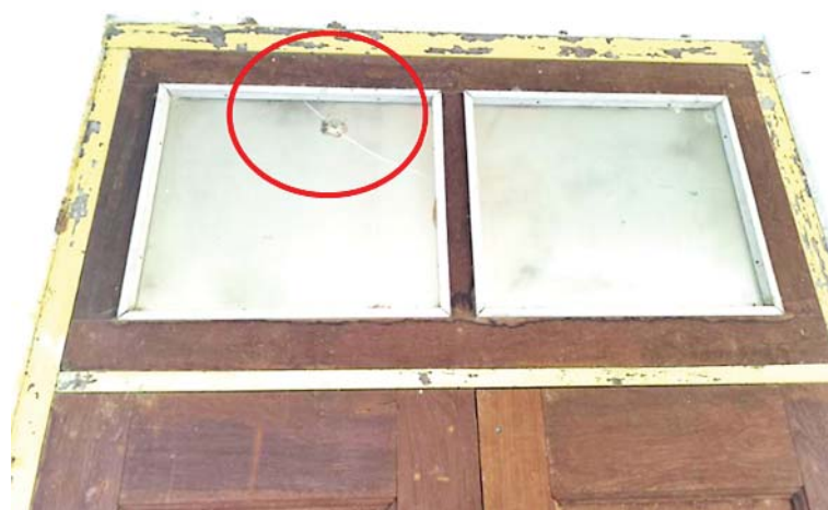
Photo shows the bullet holes caused by terrorist insurgent attack on a polling station in NyaungU, Mandalay Region.
