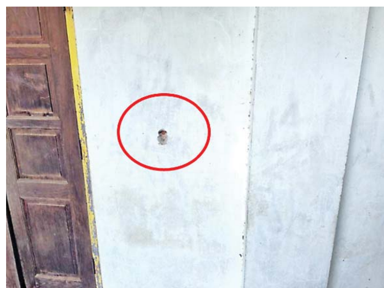
Photo shows the bullet holes caused by terrorist insurgent attack on a polling station in NyaungU, Mandalay Region.
