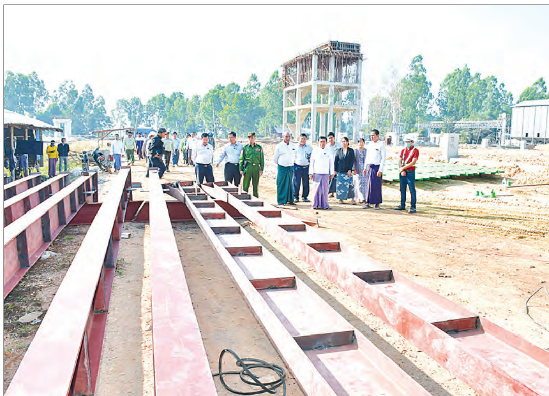
The rice bran oil and cooking oil factory under construction in Nay Pyi Taw.
