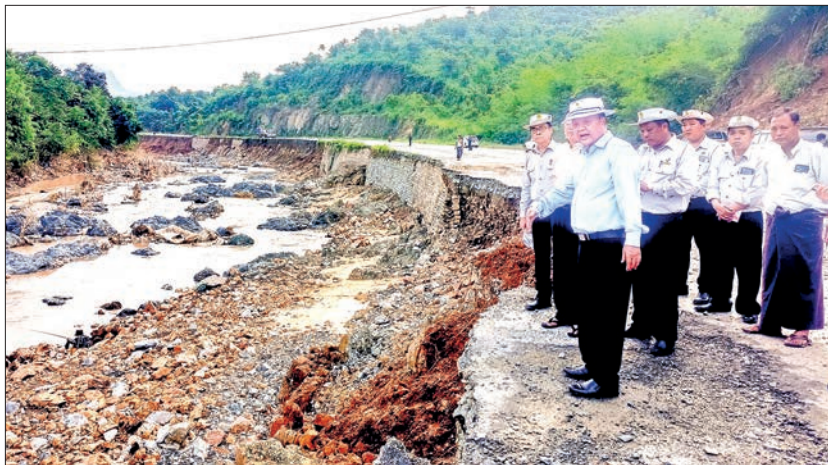
Deputy Minister U Win Pe inspects the maintenance works on the Meiktila-Taunggyi Road, which was damaged by recently torrential rainfalls.
