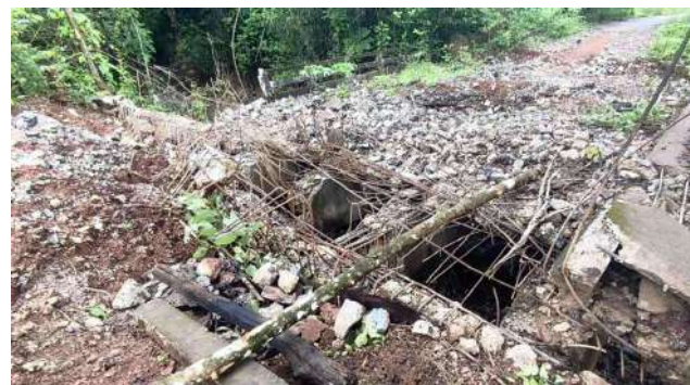
Bridge near Hpa Lon Lay village on Kamamaung–Hpapun road destroyed by terrorist insurgents.
