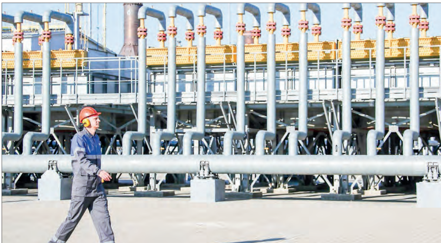
A worker walks by an air gas cooling unit at the Russkaya Compressor Station of the TurkStream gas pipeline in southern Russia’s Krasnodar region. PHOTO: DMITRY FEOKTISTOV / TASS / FILE
