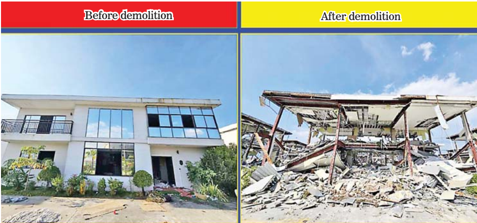
An illegally constructed two-storey residential building in Section 3 of KK Park area.
