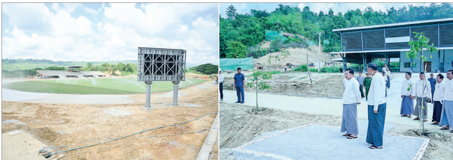
State Administration Council Chairman Prime Minister Senior General Min Aung Hlaing views the construction progress of the Naypyitaw State Polytechnic University yesterday.
