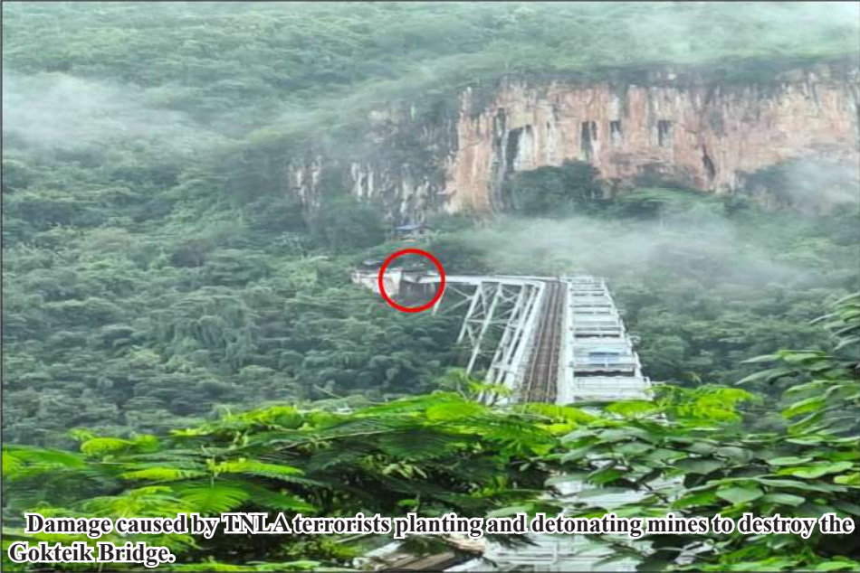
Photo record of TNLA terrorists planting and detonating mines to destroy the Gokteik Bridge.
