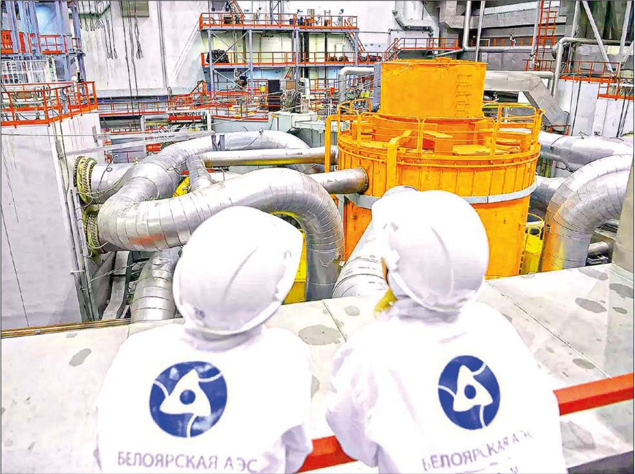
An interior view shows the Unit No 4 with the BN-800 fast reactor running on uranium-plutonium mixed-oxide (MOX) fuel at the Beloyarsk Nuclear Power Plant in Sverdlovsk Region, Russia. PHOTO: SPUTNIK
