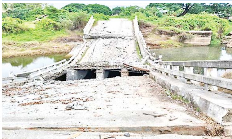
The fleeing terrorist insurgents destroyed the 55 th Mile Bridge.
