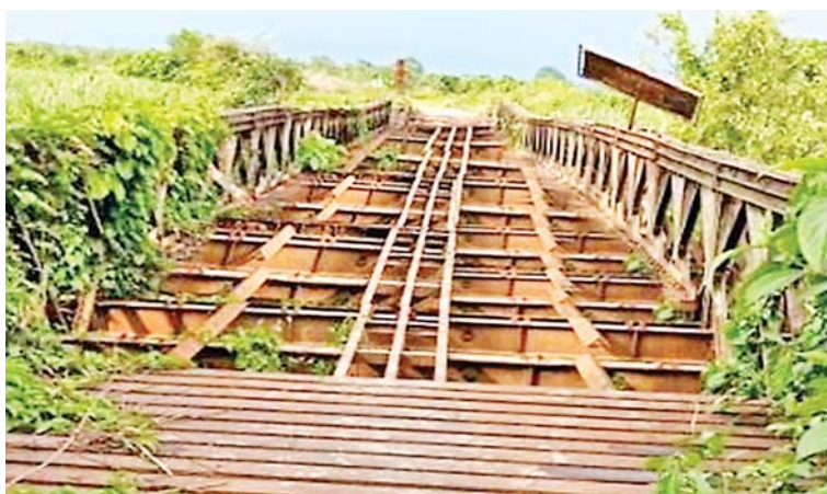
Photo shows the destroyed Nammut Bridge.
