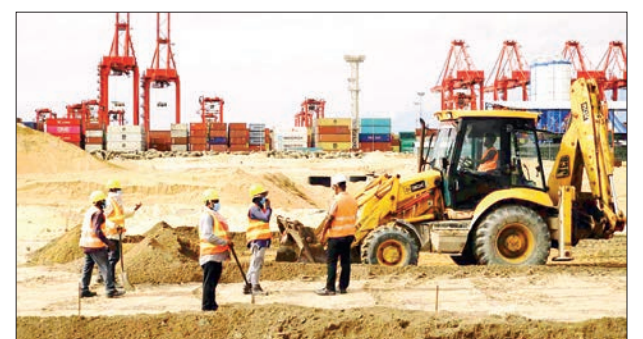
Workers undertake construction at a harbour in Colombo, Sri Lanka. PHOTO: XINHUA/FILE
