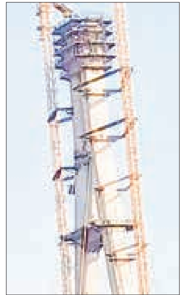
Cables are being installed in Dala, as a part of Dala-Yangon Bridge project.
