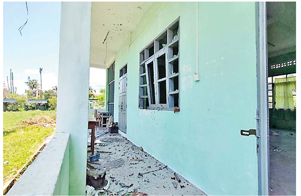
The photo shows the damage caused by terrorist drone attack.
