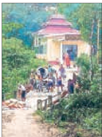
Road construction work is underway to access the mausoleum. PHOTO: THAN MIN HTUT
