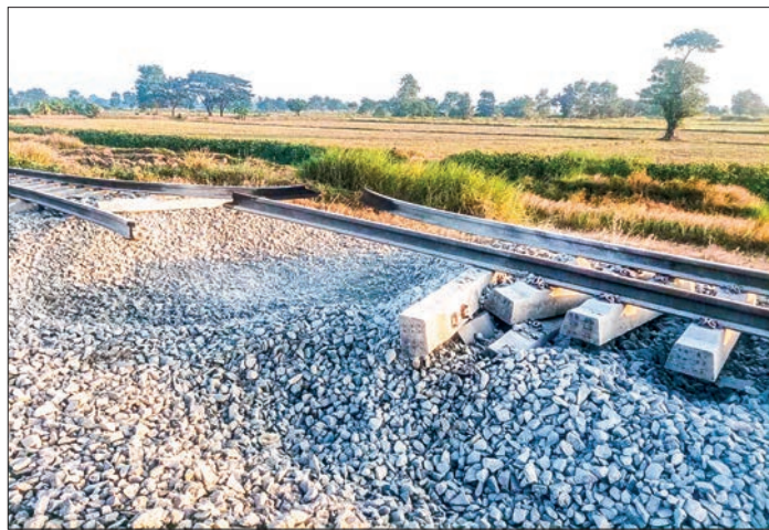
The explosion places of railway lines at mileposts 99/6-7 between Tawwi and Peinzalok stations on the Yangon-Mandalay railway destroyed by terrorists.
