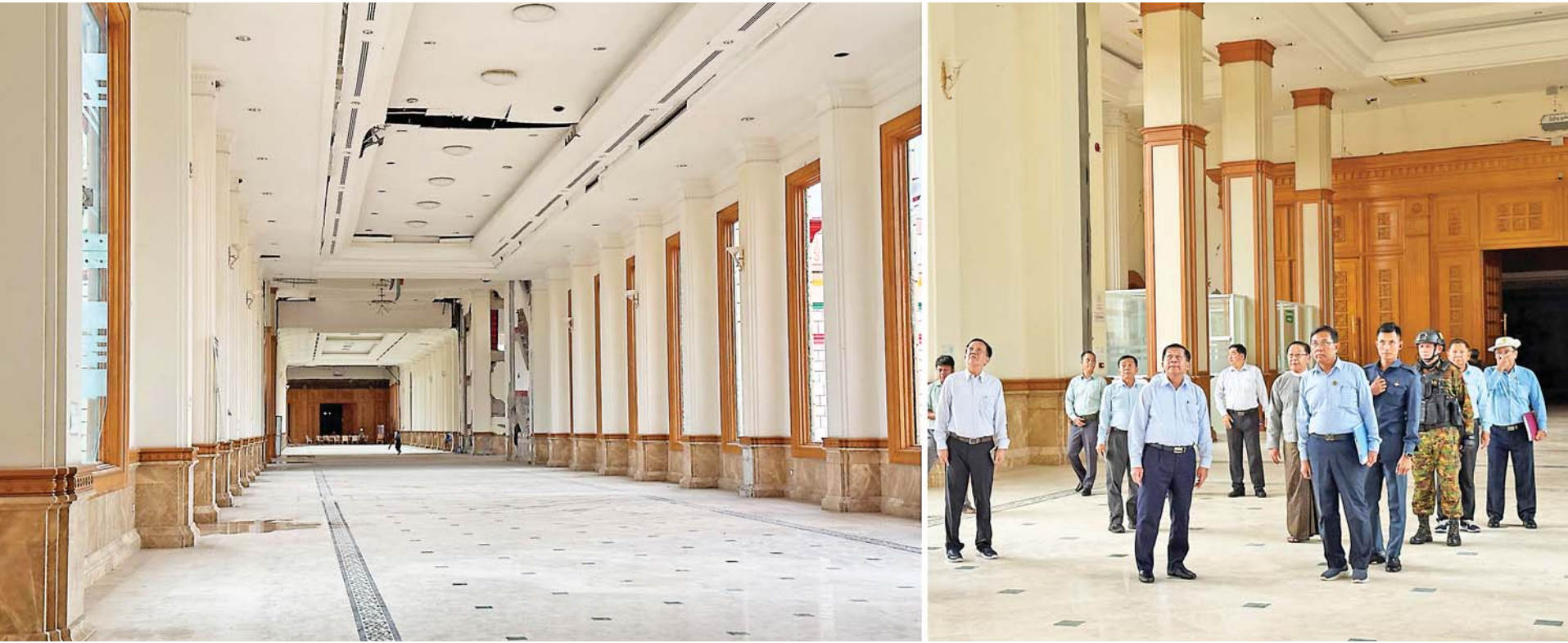
Senior General Min Aung Hlaing surveys interior damage at a Hluttaw building.
