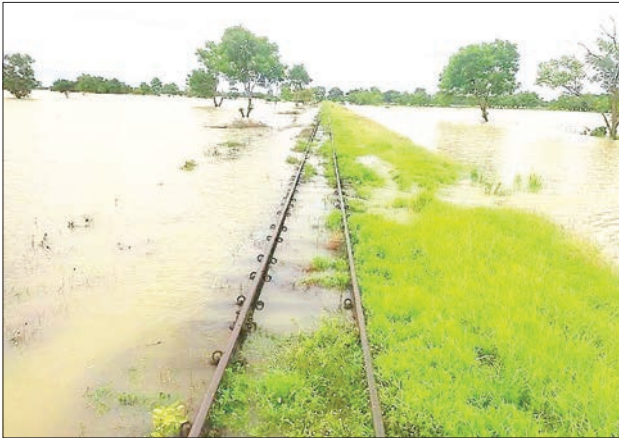
This photo captures floodwaters flowing over a section of the railway in Kyonpyaw Township, following heavy rainfall.
