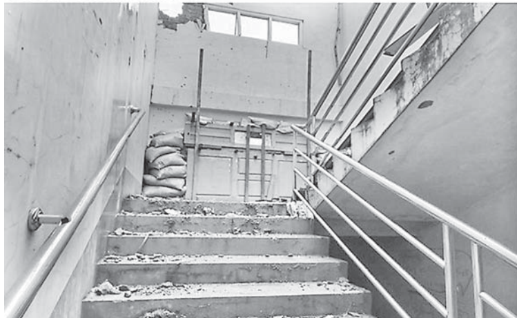
Bunkers constructed by terrorist insurgents in the Township People's Hospital in Thantlang.
