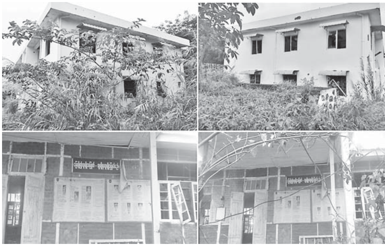
Damage to the two-storey fire services department building and the Immigration Department office buildings in Thantlang town.
