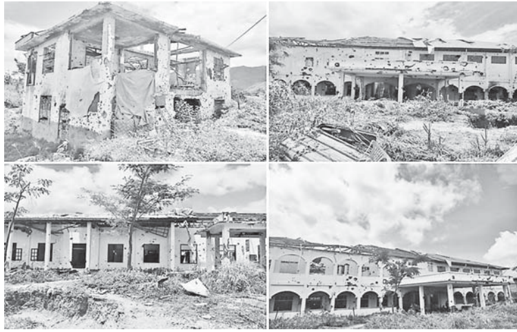
Damage to the public hospital and the Department of Religious Affairs buildings in Thantlang town.
