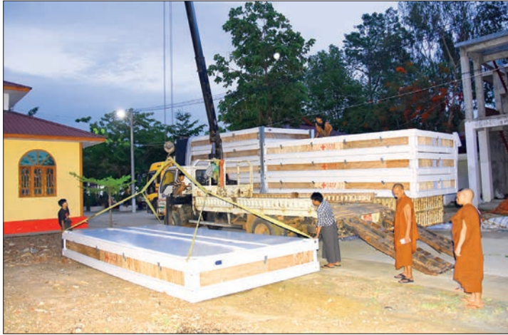
The prefabricated houses are being unload from the truck at a monastery in Nay Pyi Taw.
