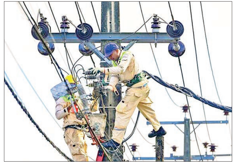
Lanka Electricity Company workers carry out maintenance work on an electric pole in Colombo, Sri Lanka in 2025. PHOTO: AFP/FILE
