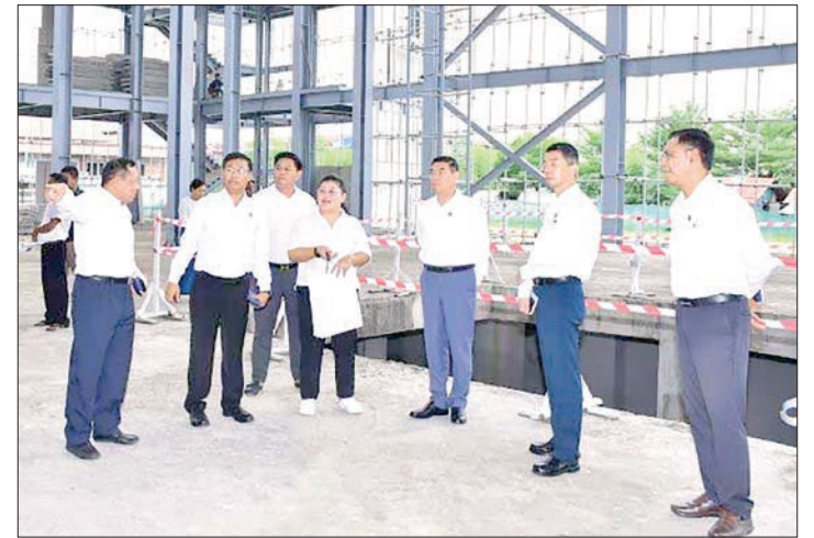
Union Minister for Information U Htein Lin inspects the progress of the construction of the Arts Centre (Mandalay) yesterday.
