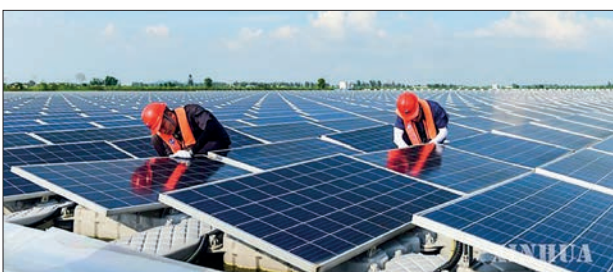
Solar panels are being installed at the power station to generate electricity in Guizhou Province, southwest China. PHOTO: XINHUA
