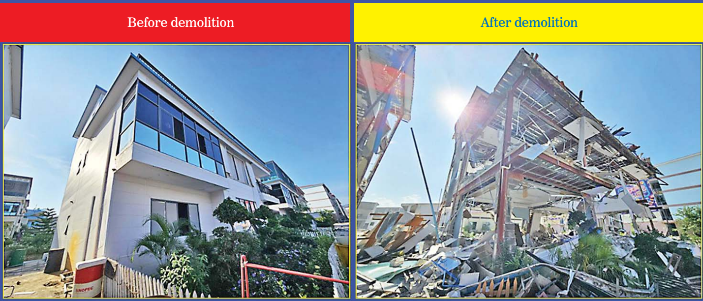
An illegally constructed three-storey building in the KK Park area part-3.
