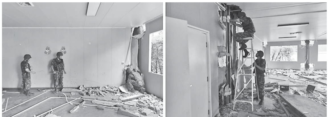
An illegal seven-story residential building used for online scam gambling operations in the Shwe Kokko Area of Myawady District, Kayin State, is being prepared to be blasted and destroyed with explosives.
